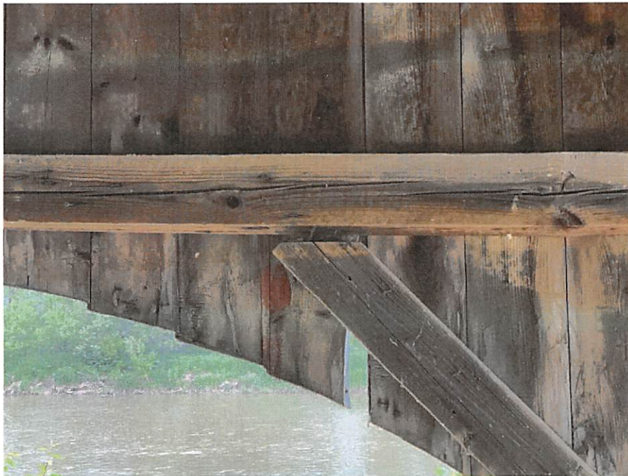
Figure 8: Gap at Knee Brace
