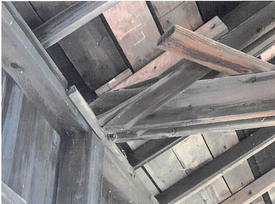
Figure 6: Crushing at Truss Bearing
