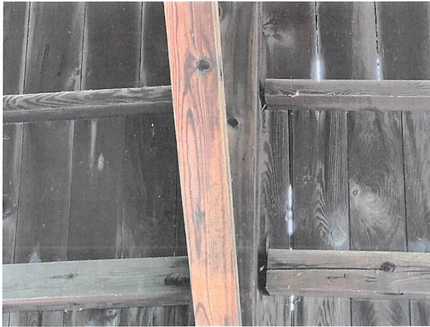
Figure 7: Gaps at Wall Girts
