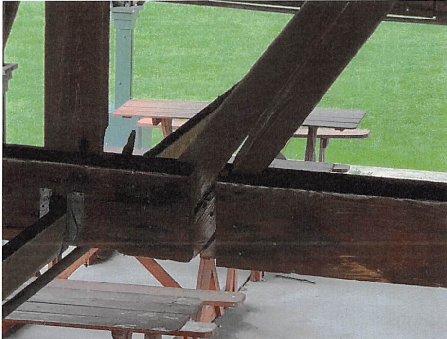
Figure 5: Split Truss Bottom Chord
